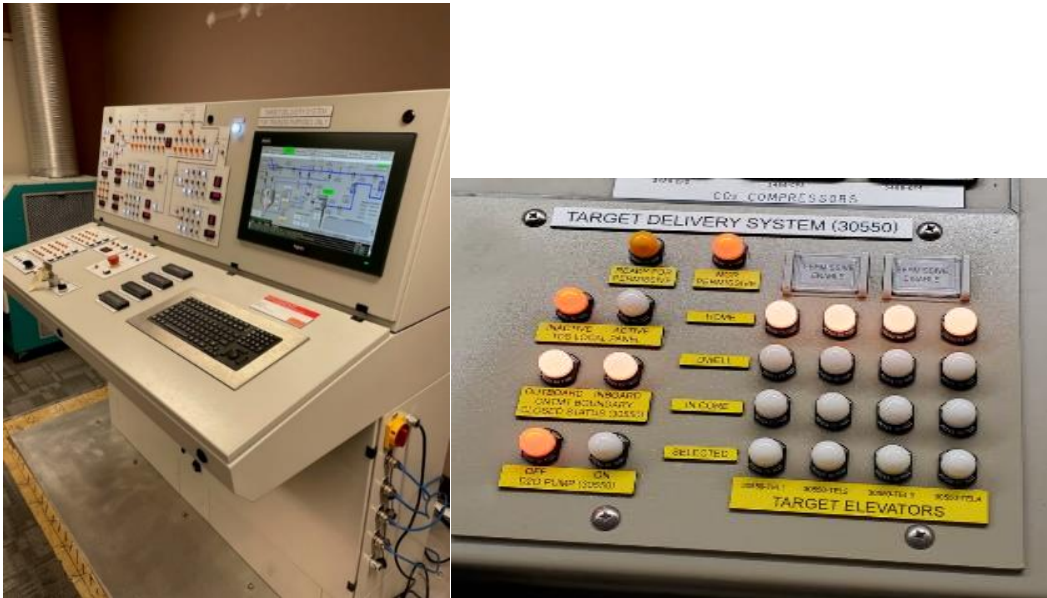
Figure 5. Field Control Panel Simulator and Main Control Room Simulator Interface
